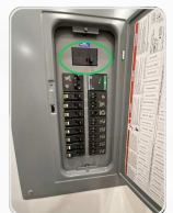
PHOTO — MAIN DISCON
