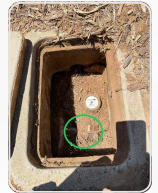
PHOTO — WATER UTILITY
